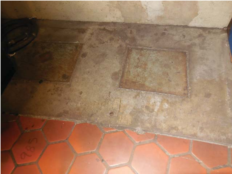
Pictures 1&2: C02 McPherson Sq (East) – Handholes in mezzanine
