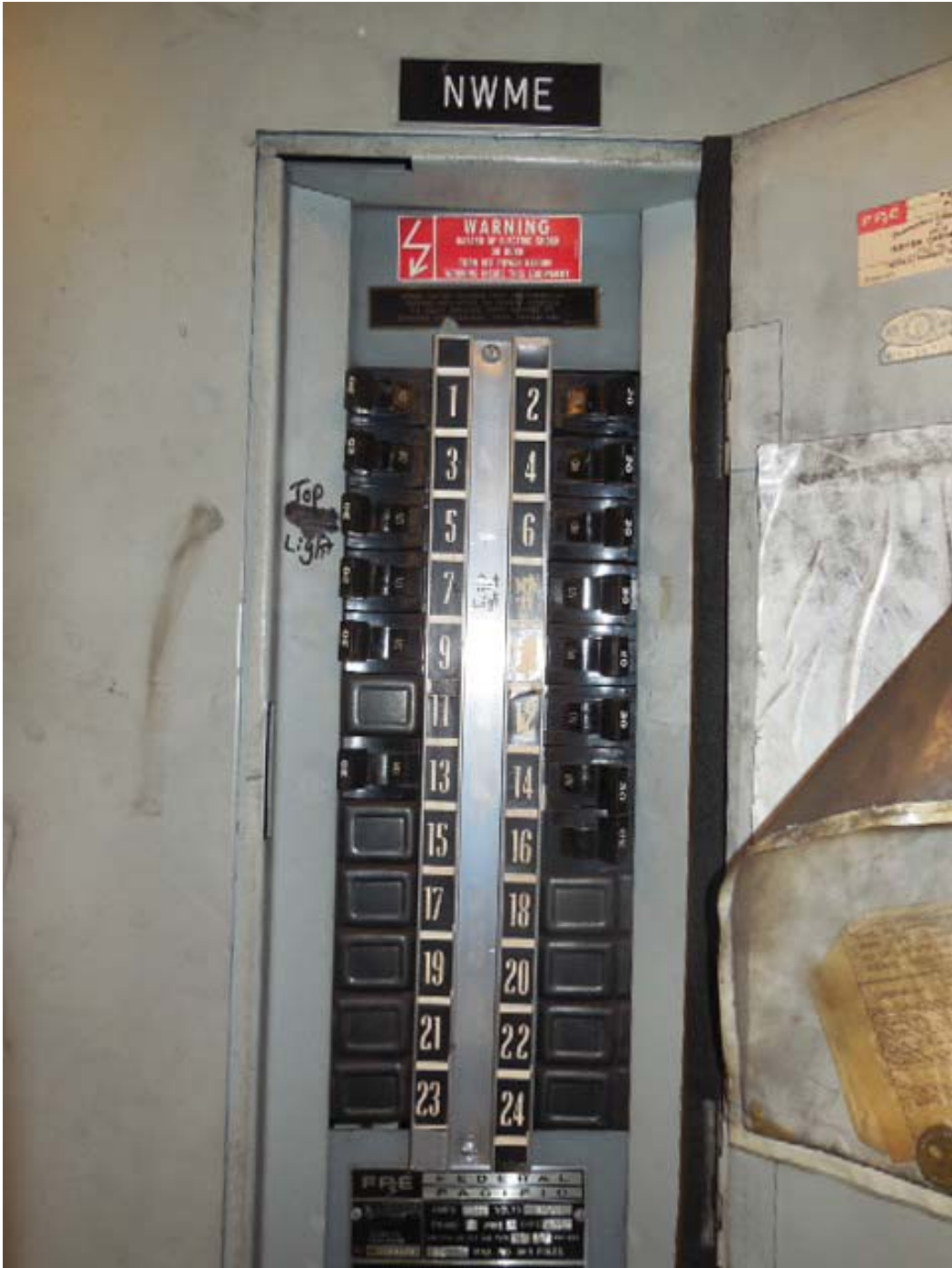
Picture 12: C02 McPherson Sq (West) – Emergency Panel NWME in room 212
