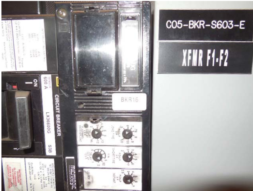
Picture 3: C05 Rosslyn – SWBD breaker for XFMR F1-F2 in room 112
