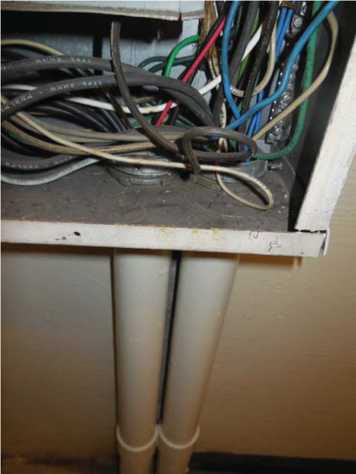
Picture 9: C06 Arlington Cemetery – AFC Panel F-1 in Room 100 – Conduits below panel
