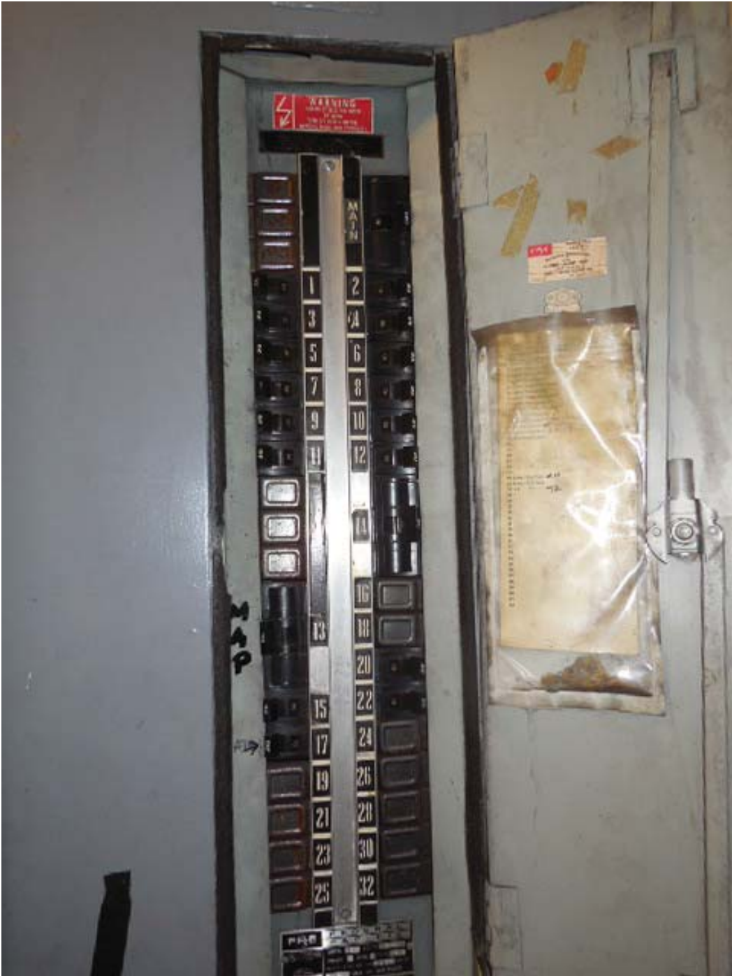
Picture 16: C04 Foggy Bottom – AFC Panel 2MM in room C204
