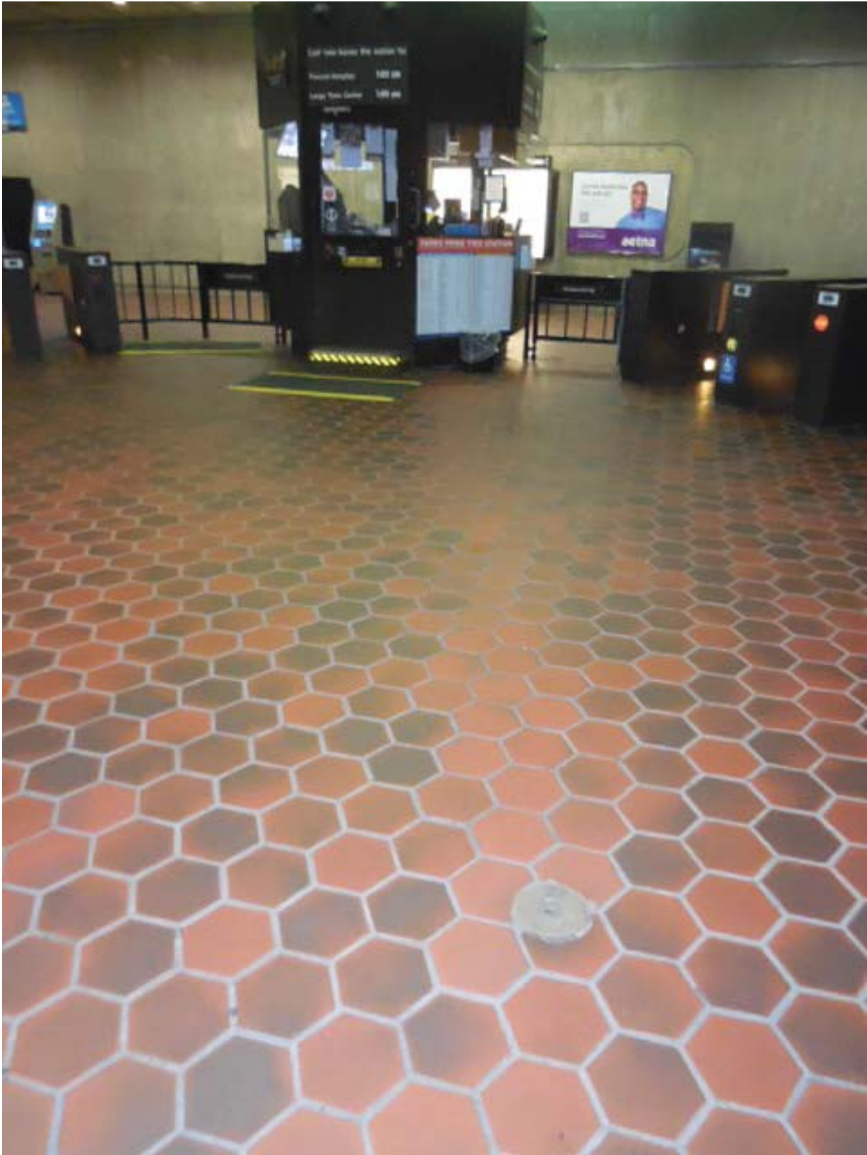
Picture 1: C06 Arlington Cemetery – Handholes in Mezzanine
