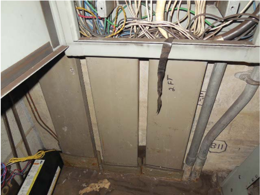
Picture 9: C05 Rosslyn (NEW) – AFC Panel F1 in room W110, Ducts below panel
