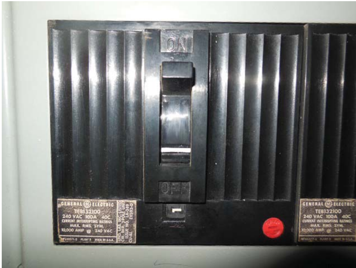
Picture 14: C06 Arlington Cemetery – North Dist. Panel in Room C206 – Breaker 1
