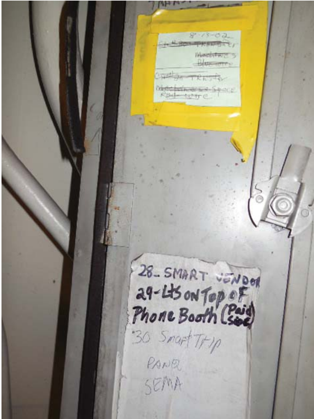
Picture 8: C03 Farragut West – AFC Panel SEMA in Rm 201, panel schedule
