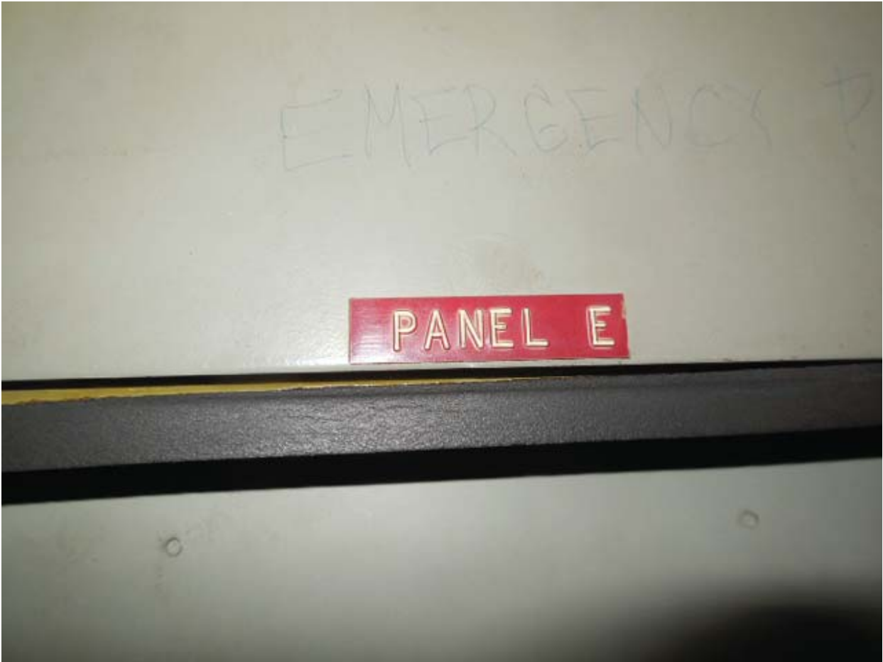
Picture 11: C06 Arlington Cemetery – Emergency Panel E in Room C206
