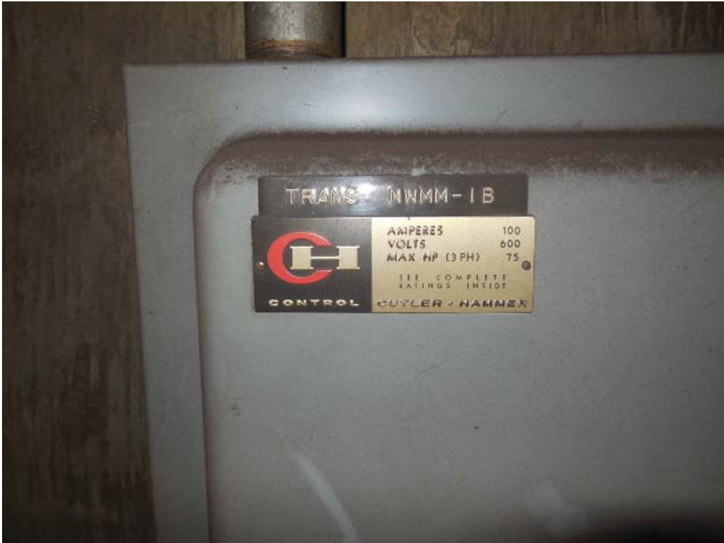
Picture 10: C02 McPherson Sq (West) – Transformer for AFC Panel NWMM-1B in room 212
