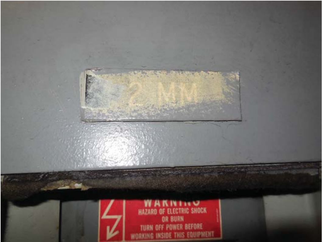
Picture 15: C04 Foggy Bottom – AFC Panel 2MM in room C204
