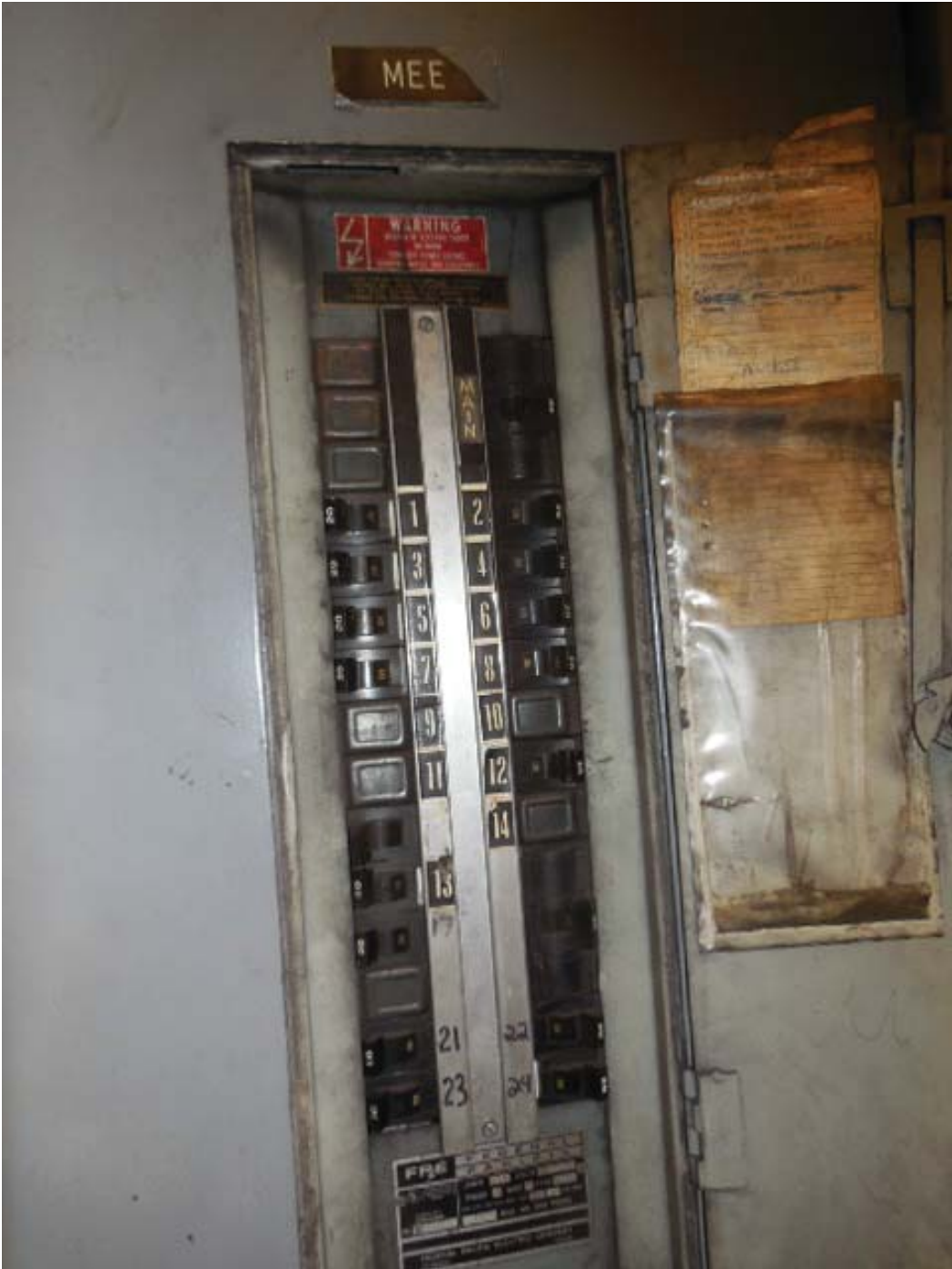
Picture 20: C04 Foggy Bottom – Emergency Panel MEE in room C204
