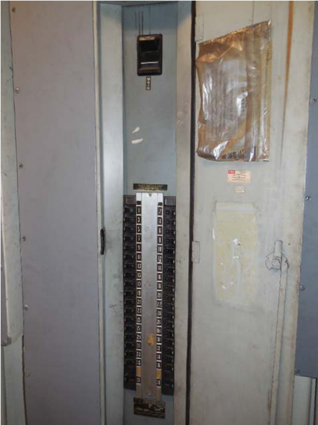
Picture 12: C04 Foggy Bottom – AFC Panel 1MM in room C204
