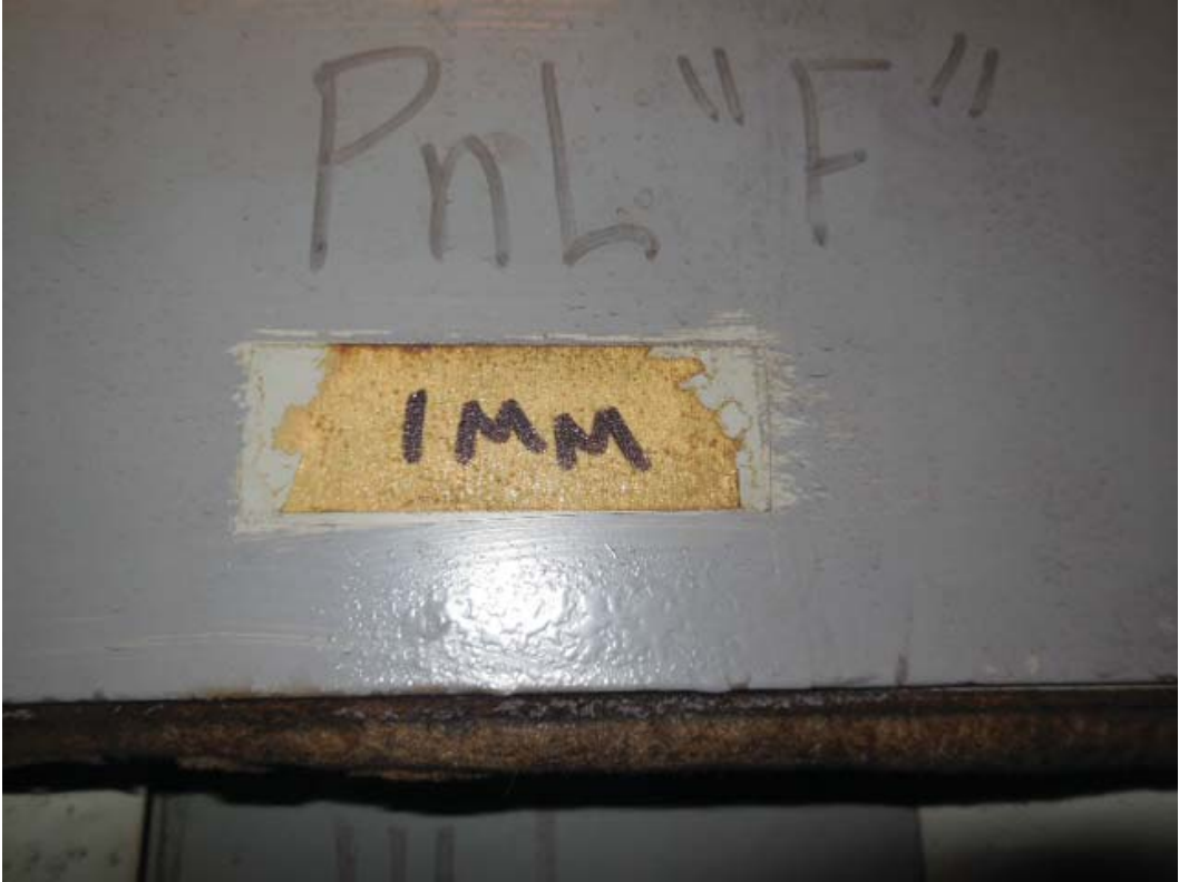
Picture 11: C04 Foggy Bottom – AFC Panel 1MM in room C204
