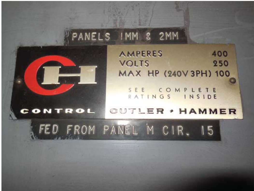
Picture 18: C04 Foggy Bottom – Disconnect Switch ‘PANELS 1MM & 2MM FED FROM PANEL M CIR.15’
