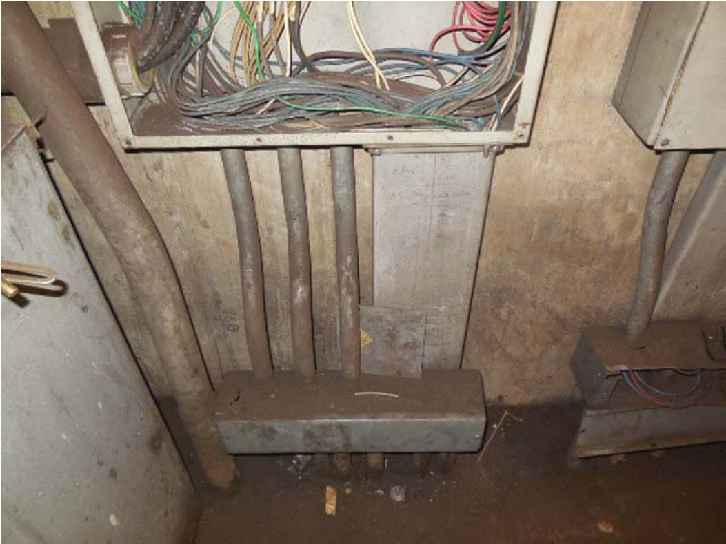
Picture 9: C02 McPherson Sq (West) - AFC Panel NWMM-1B in room 212 – Bottom duct and conduits
