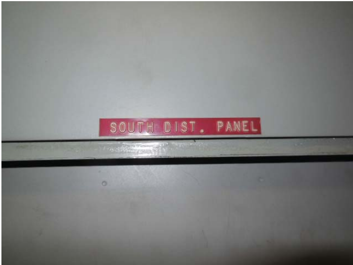
Picture 16: C06 Arlington Cemetery – South Dist. Panel in Room C206
