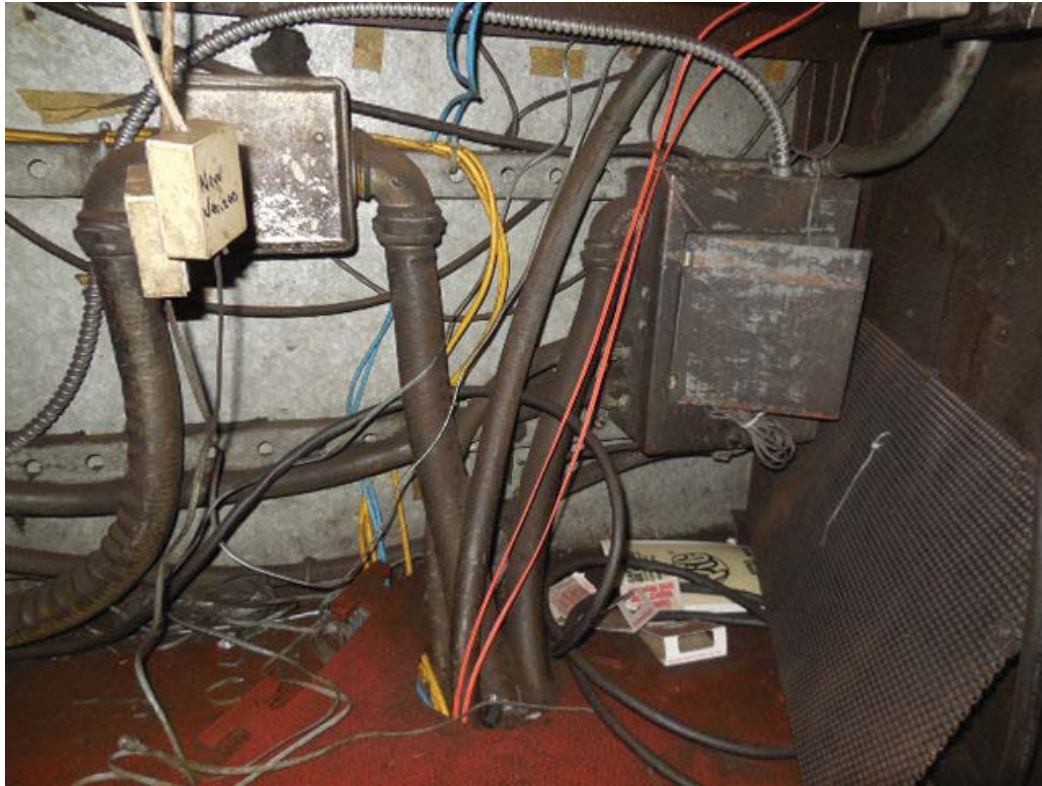
Pictures 4&5: C02 McPherson Sq (West) – Emergency panel in Kiosk
