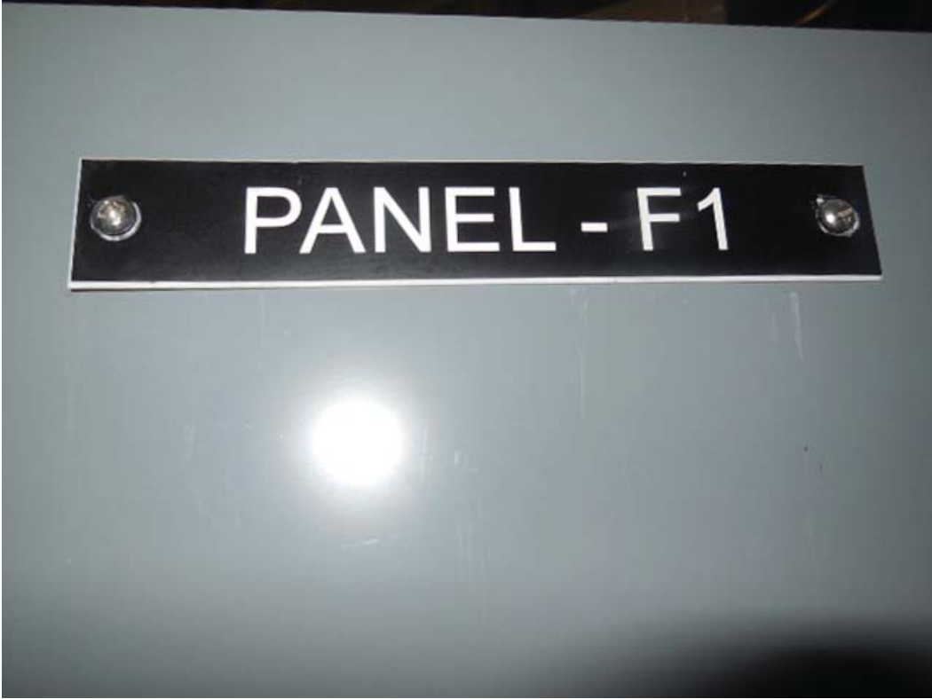
Picture 7: C05 Rosslyn (NEW) – AFC Panel F1 in room W110
