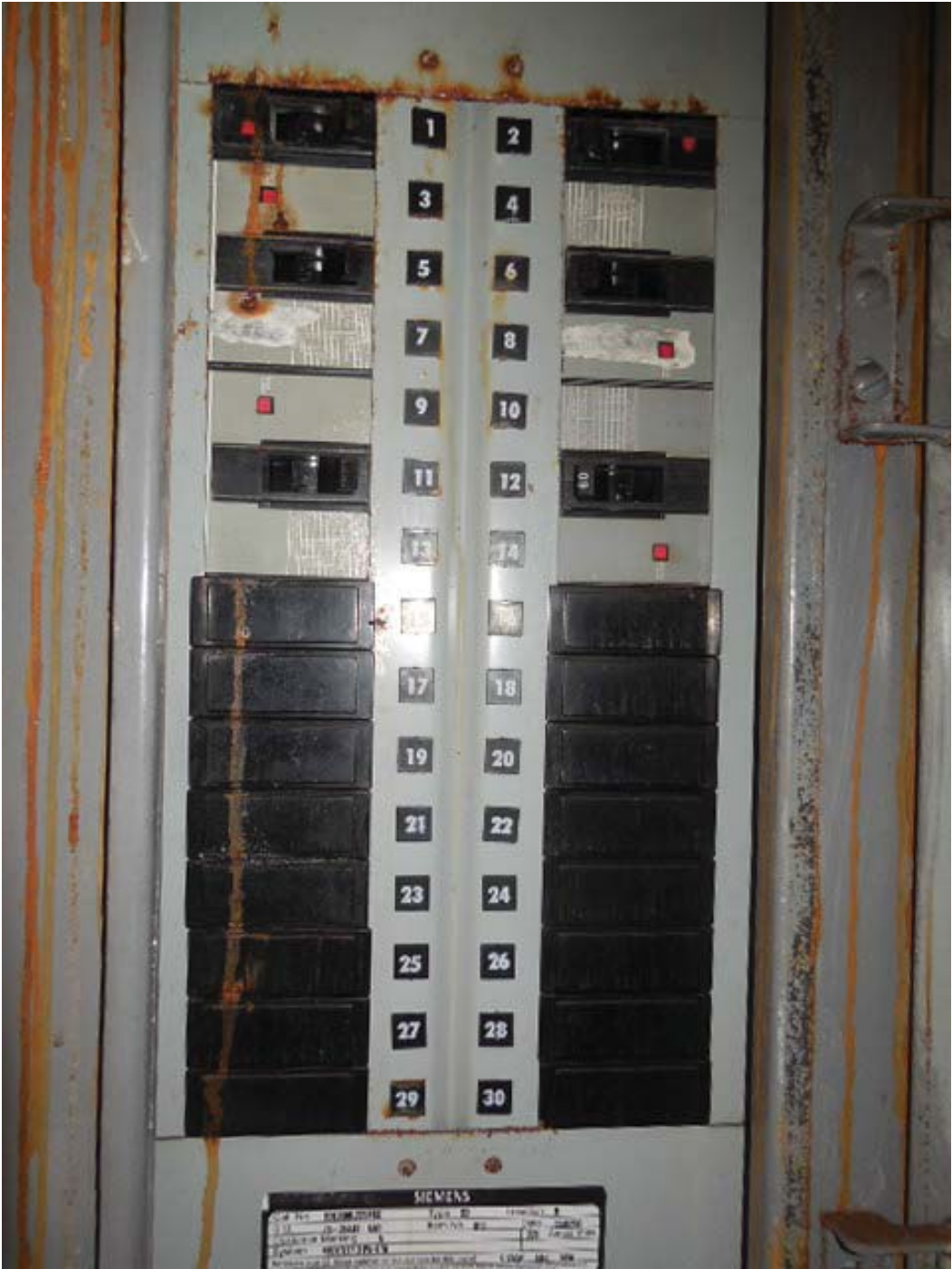
Picture 9: C03 Farragut West – Panel SEPOA in Rm 201
