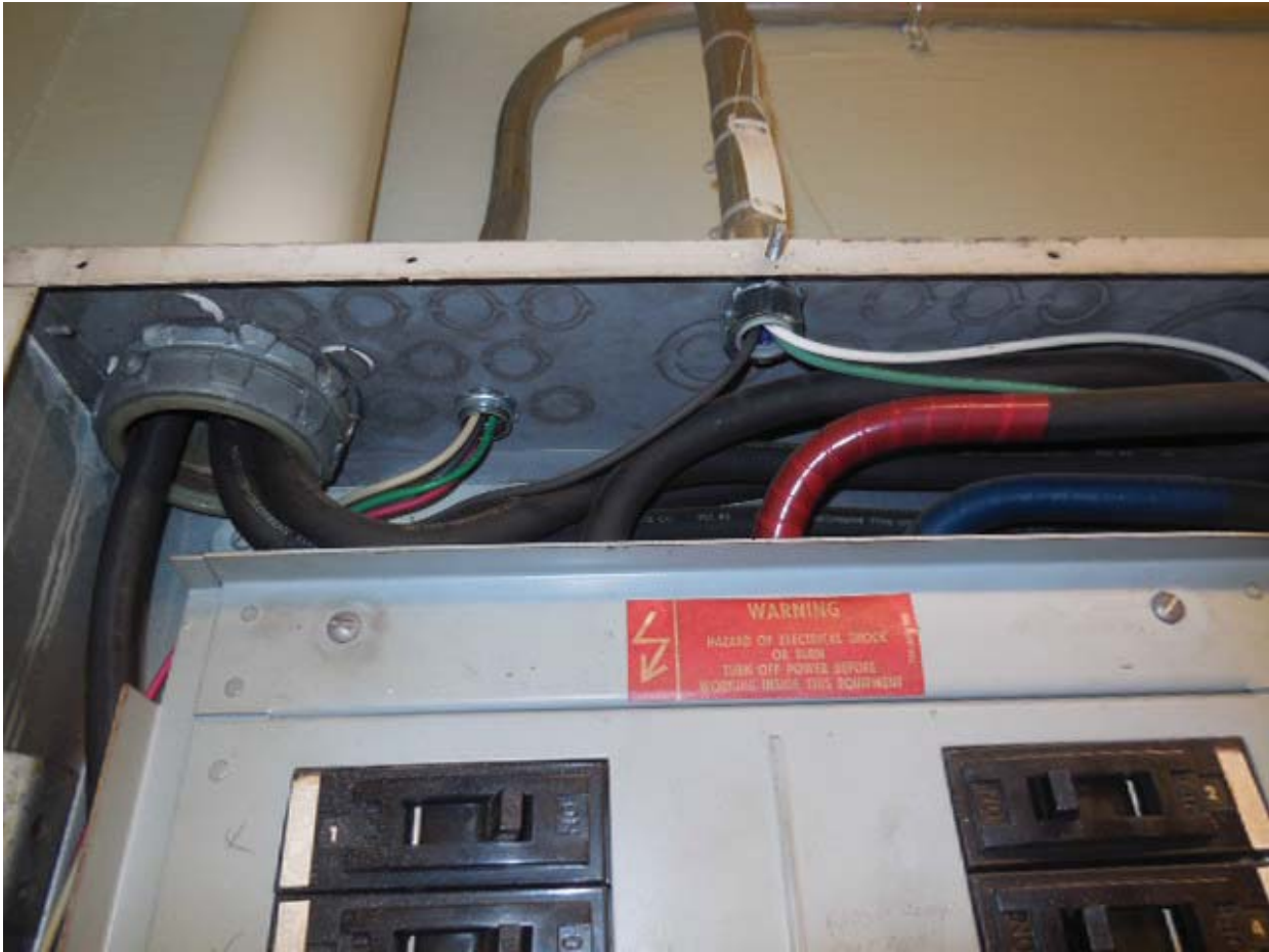
Picture 8: C06 Arlington Cemetery – AFC Panel F-1 in Room 100 – Conduits above panel
