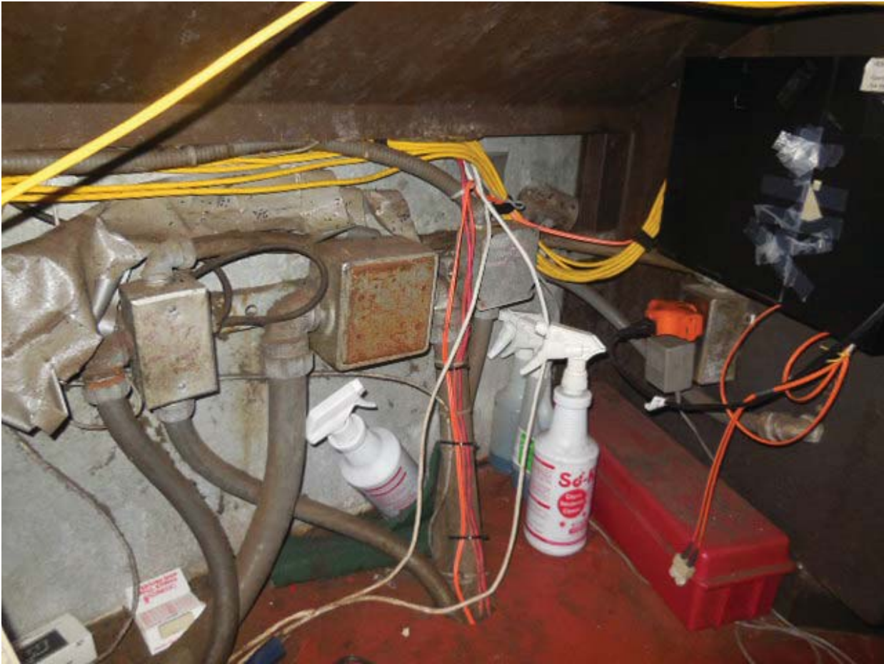
Pictures 4: C06 Arlington Cemetery – Emergency panel in Kiosk
