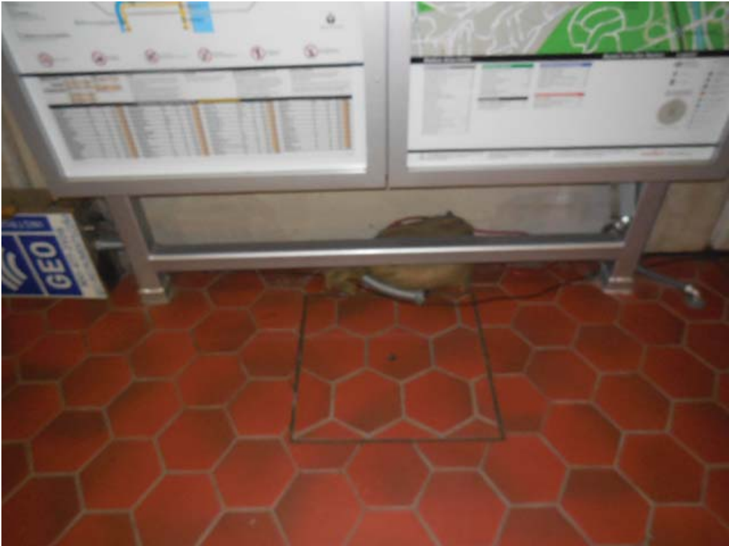
Picture 3: C05 Rosslyn (NEW) – Handholes in mezzanine
