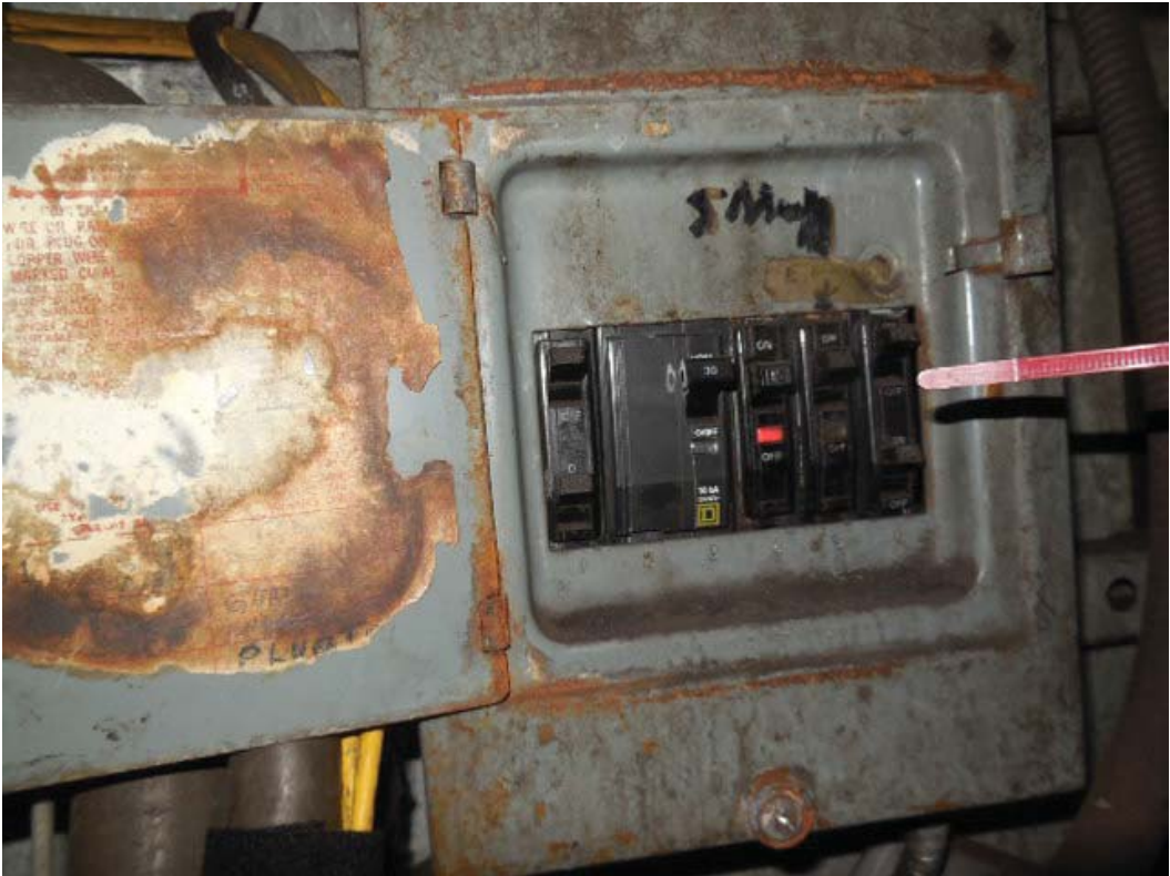
Pictures 4&5: C02 McPherson Sq (East) – Emergency panel in Kiosk
