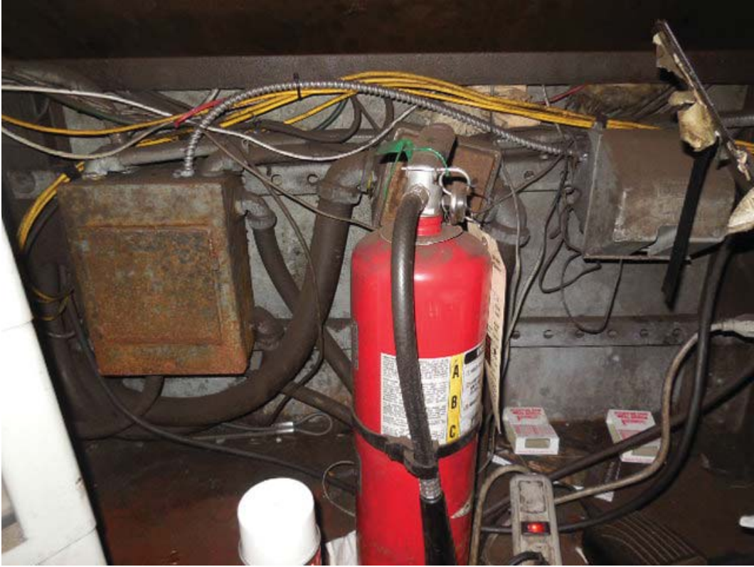
Pictures 8&9: C04 Foggy Bottom – Emergency panel in Kiosk
