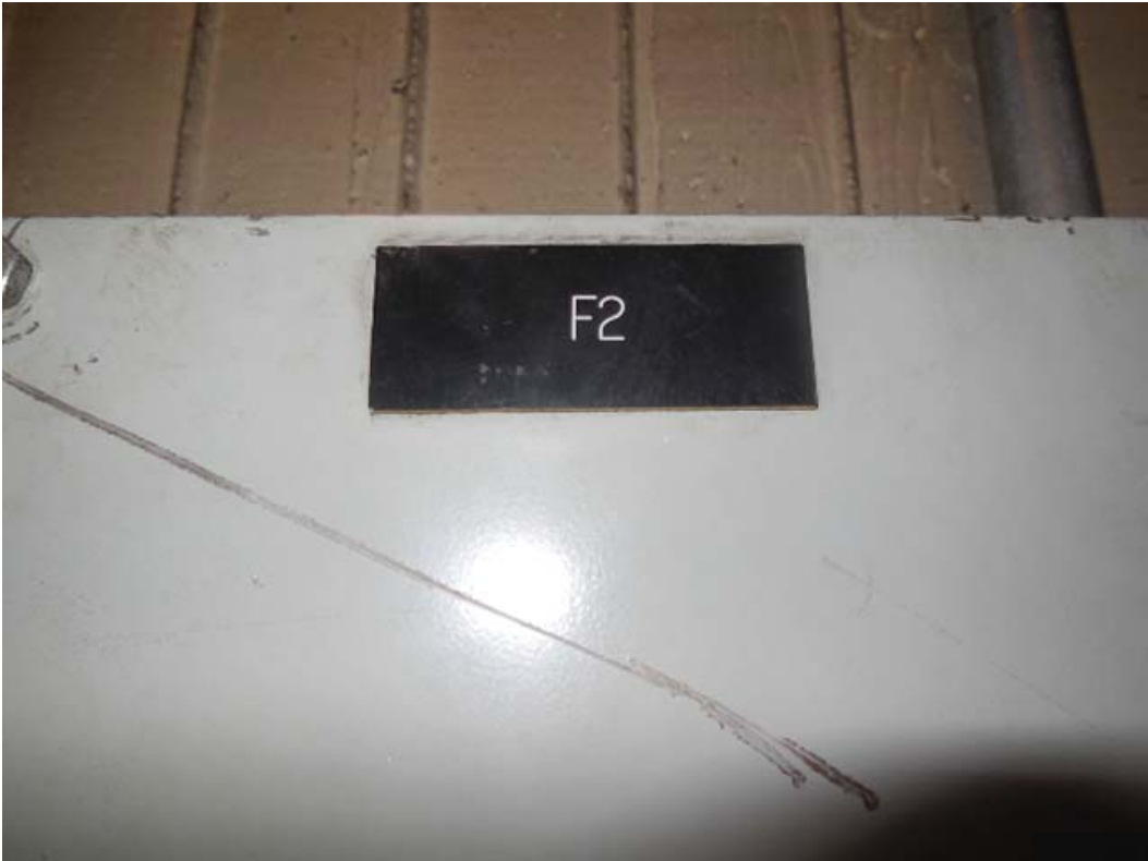
Picture 4: C05 Rosslyn – AFC Panel F2 in room C304
