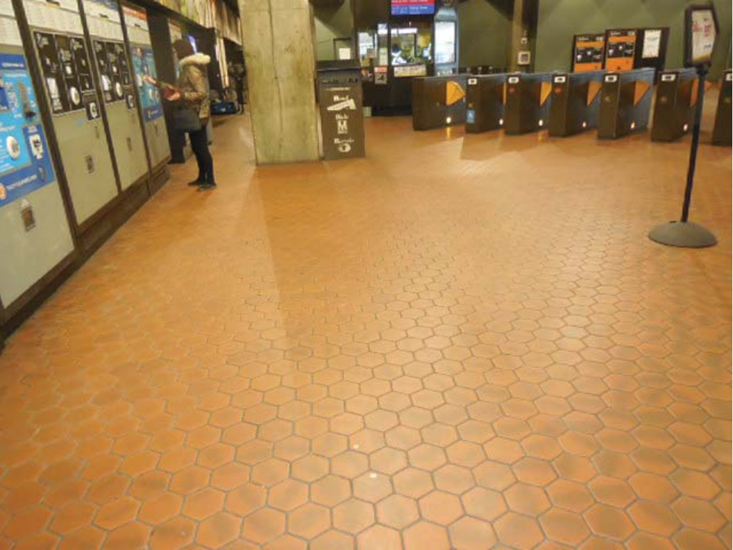
Picture 2: C05 Rosslyn – No handholes in mezzanine on free side
