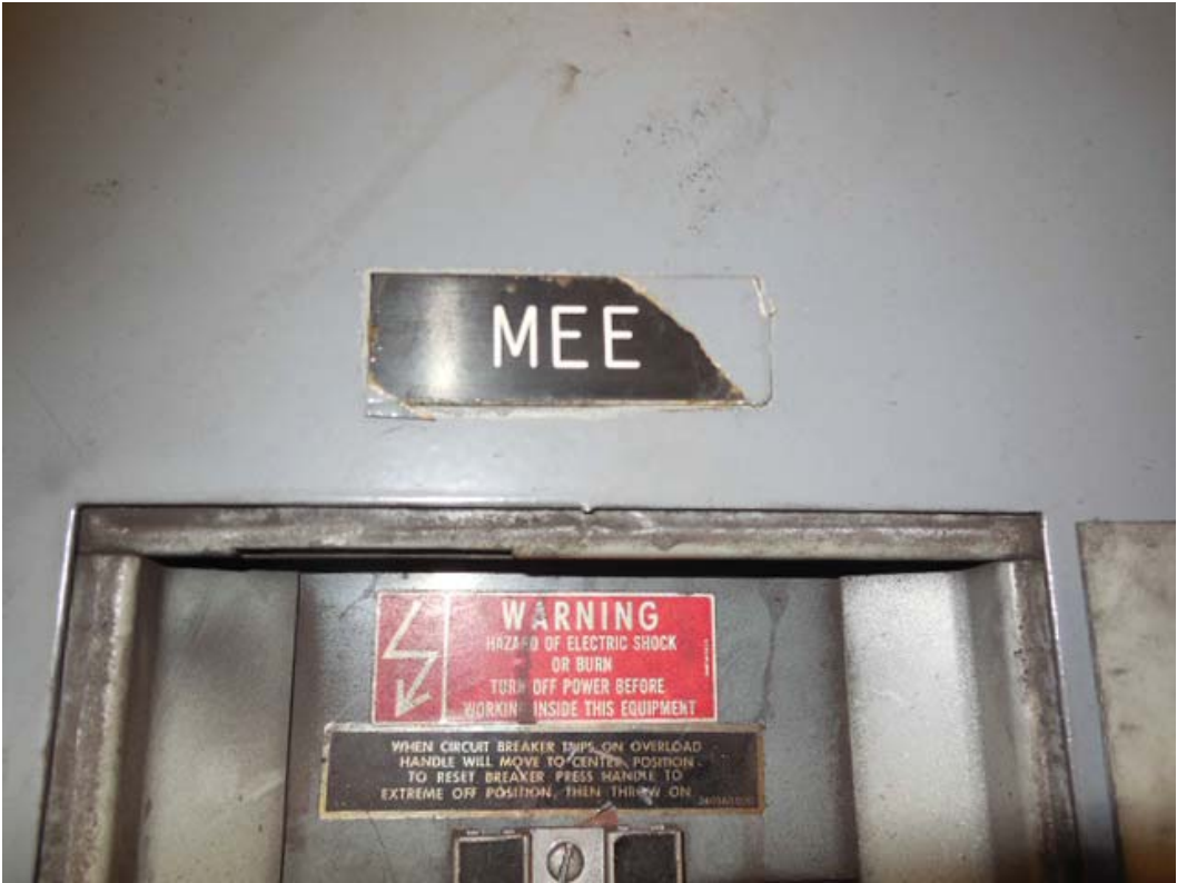
Picture 19: C04 Foggy Bottom – Emergency Panel MEE in room C204
