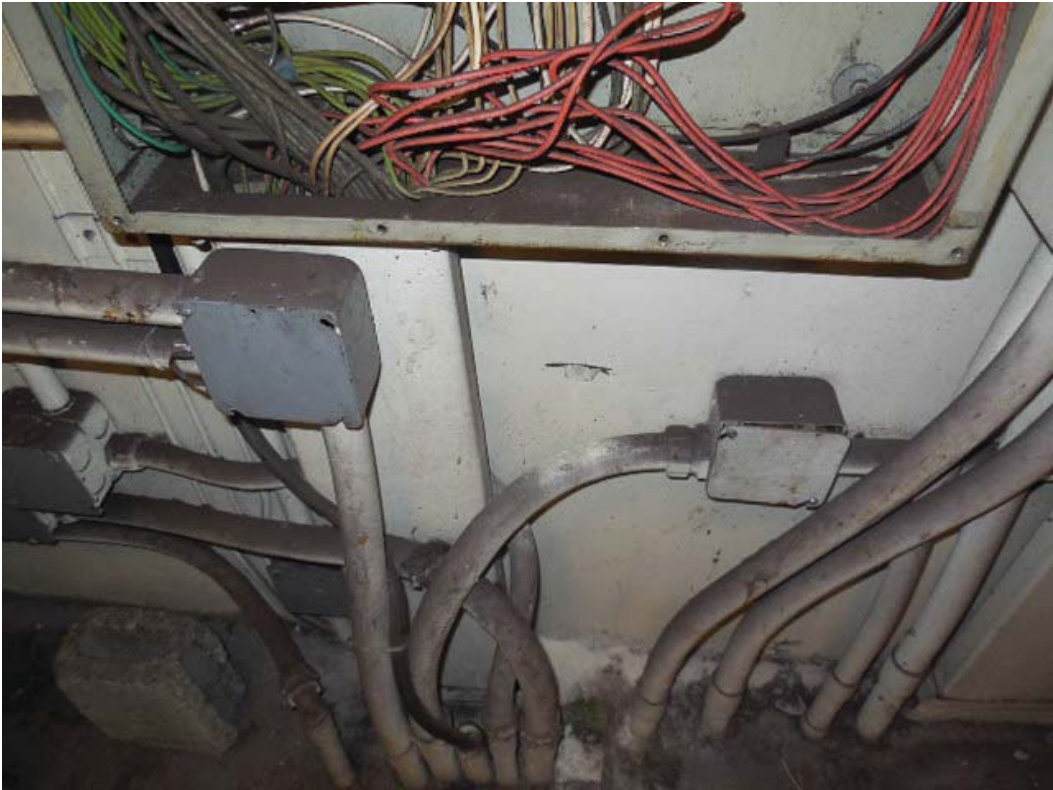
Picture 8: C02 McPherson Sq (East) – AFC Panel NEMM-IB in room 211 – Bottom duct
