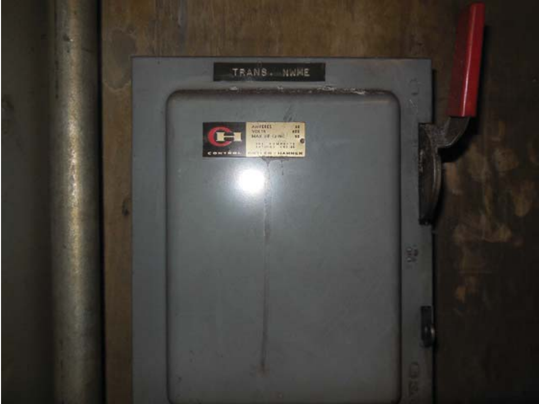
Picture 11: C02 McPherson Sq (West) – Disconnect switch for Trans NWMM-1B in room 212
