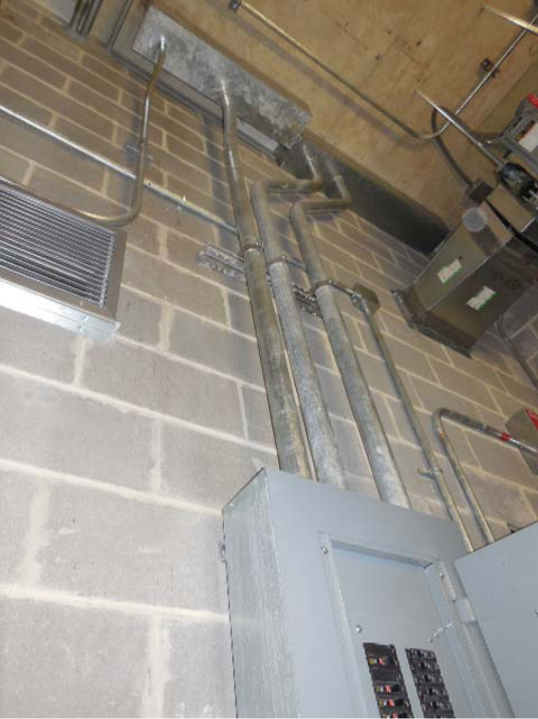
Picture 8: C05 Rosslyn (NEW) – AFC Panel F1 in room W110, Conduits and troughs above panel
