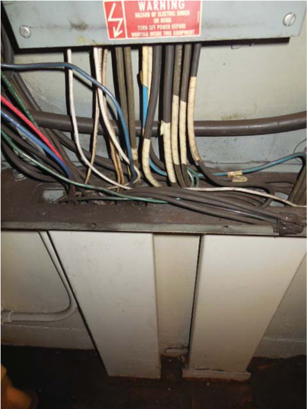
Picture 7: C03 Farragut West – AFC Panel SEMA in Rm 201, bottom ducts
