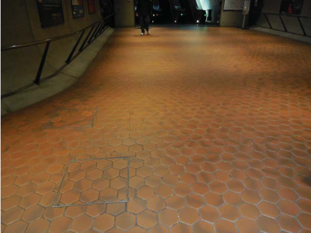
Pictures 1&2: C03 Farragut West – Handholes in mezzanine
