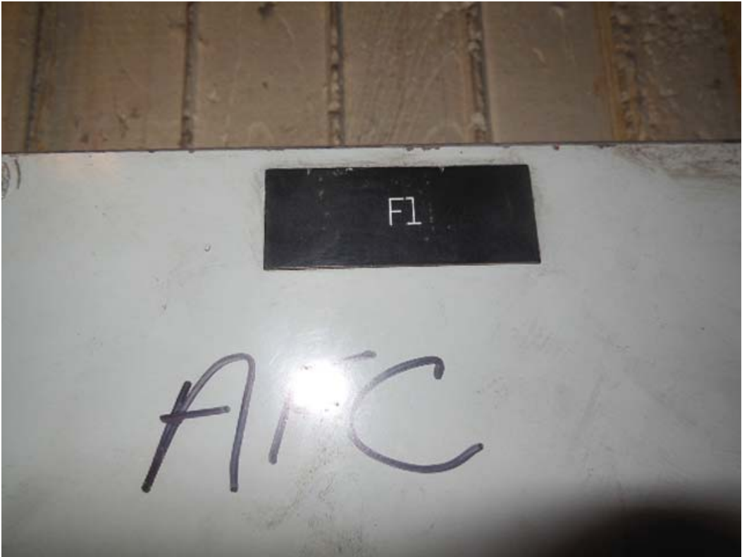
Picture 6: C05 Rosslyn – AFC Panel F1 in room C304
